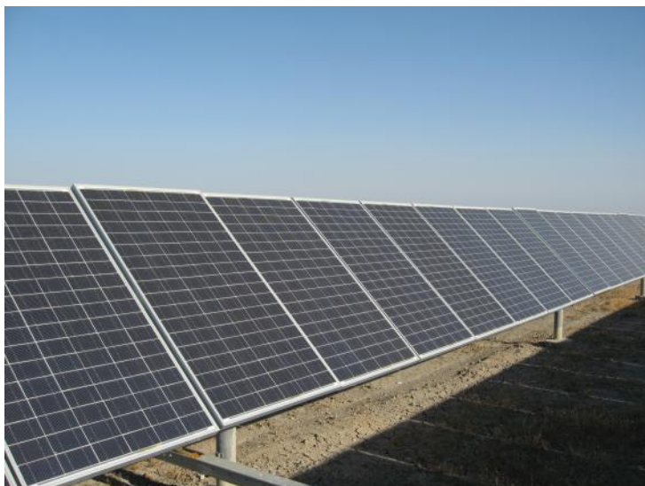
Figure 2.2: Photograph illustrating photovoltaic panels
