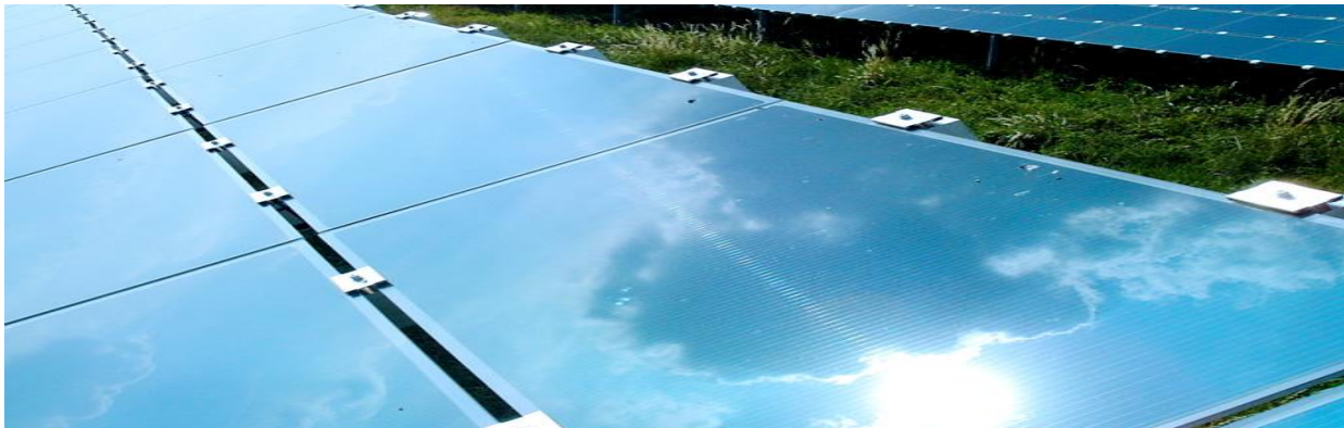
Figure 5. Close up of a Solar Photovoltaic Panel
