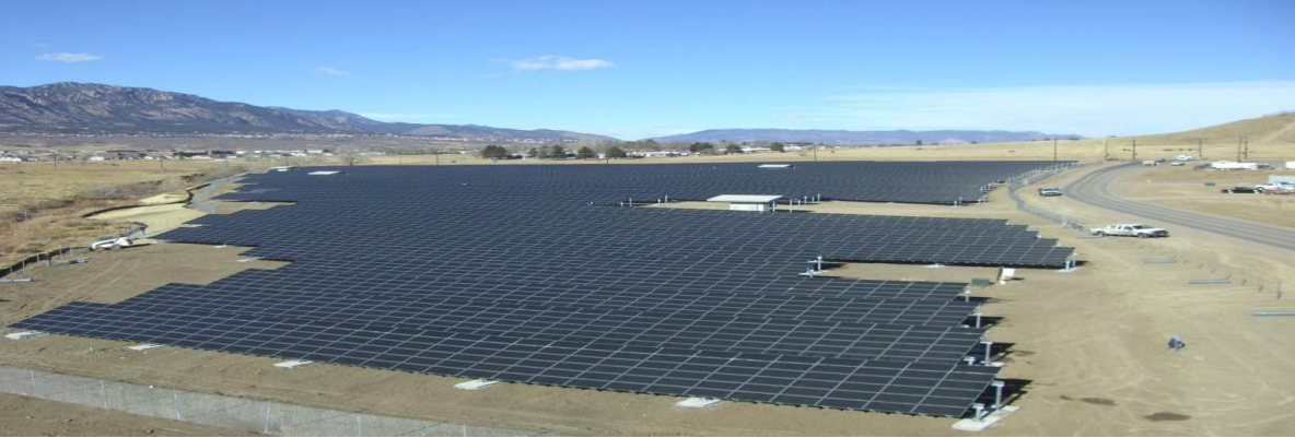
Figure 6. Large scale Solar PV array
