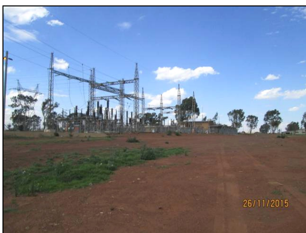
The Eskom substation partially located on site.
