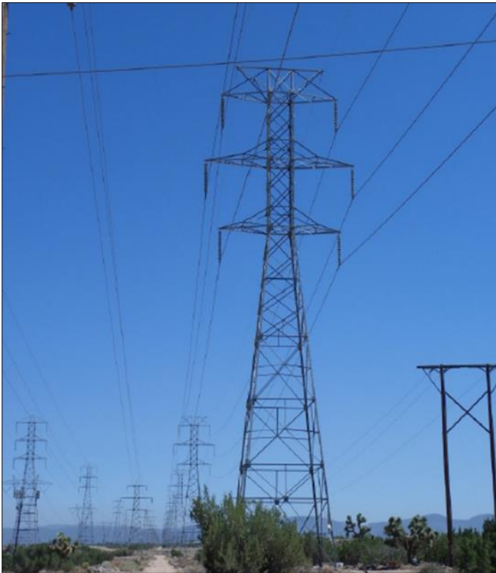
Figure 5-5: 132KV/275KV Powerline Double Circuit Suspension Towers
