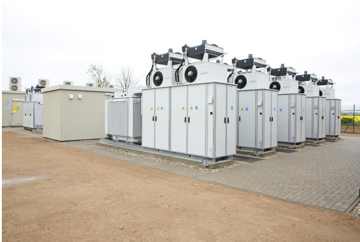
Figure 2.4: Li-Ion BESS containerised modules located within the BESS enclosure footprint (Source: Enel Green Power).
