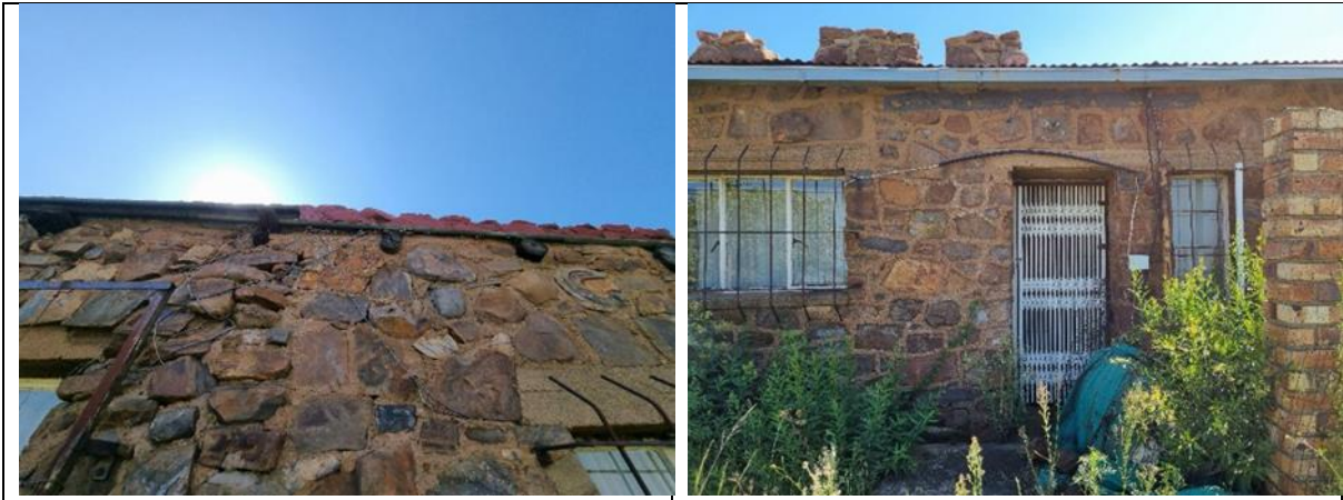
Figure 10.4-37 : Farm outbuilding. Likely livestock pen/chicken coop. Left, south facing wall; Right west facing wall.
