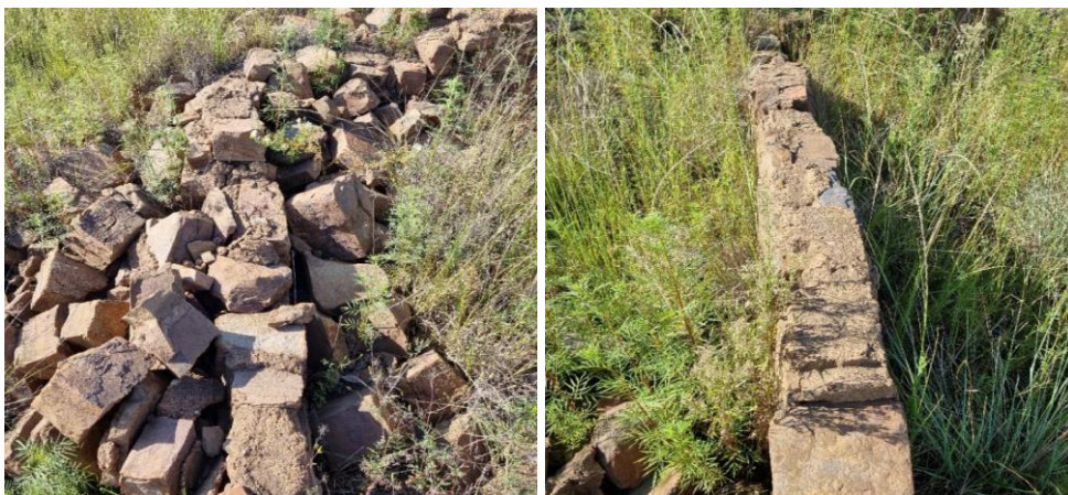
Figure 10.4-51 : Collapsed free standing brick and cement walls. UP-DRB-2529-06 (left) and UP-DRB-2529-07 (right).
