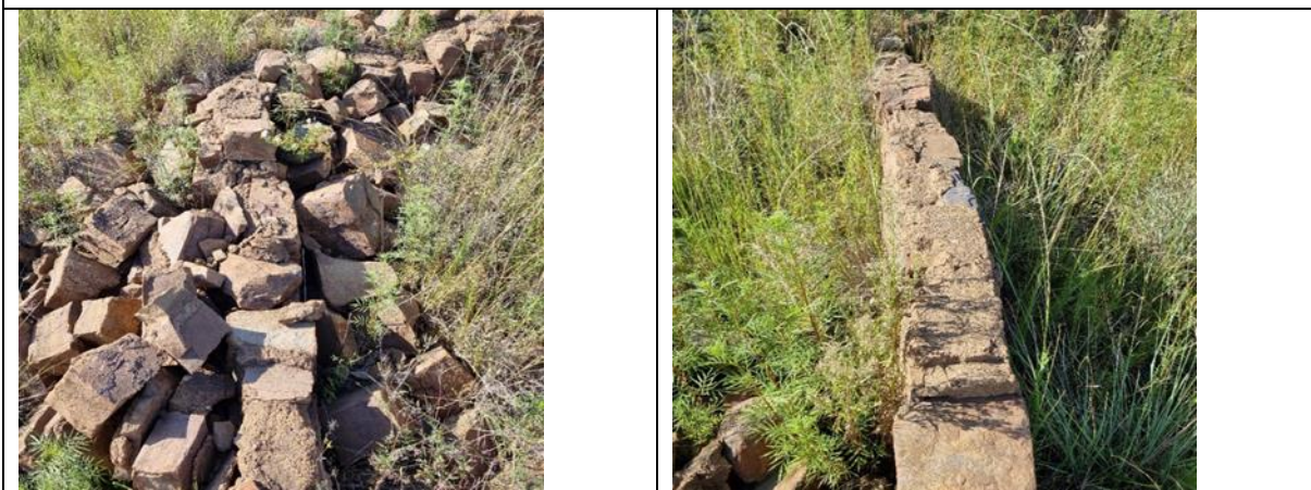
Figure 8-51 : Collapsed free standing brick and cement walls. UP-DRB-2529-06 (left) and UP-DRB-2529-07 (right).
