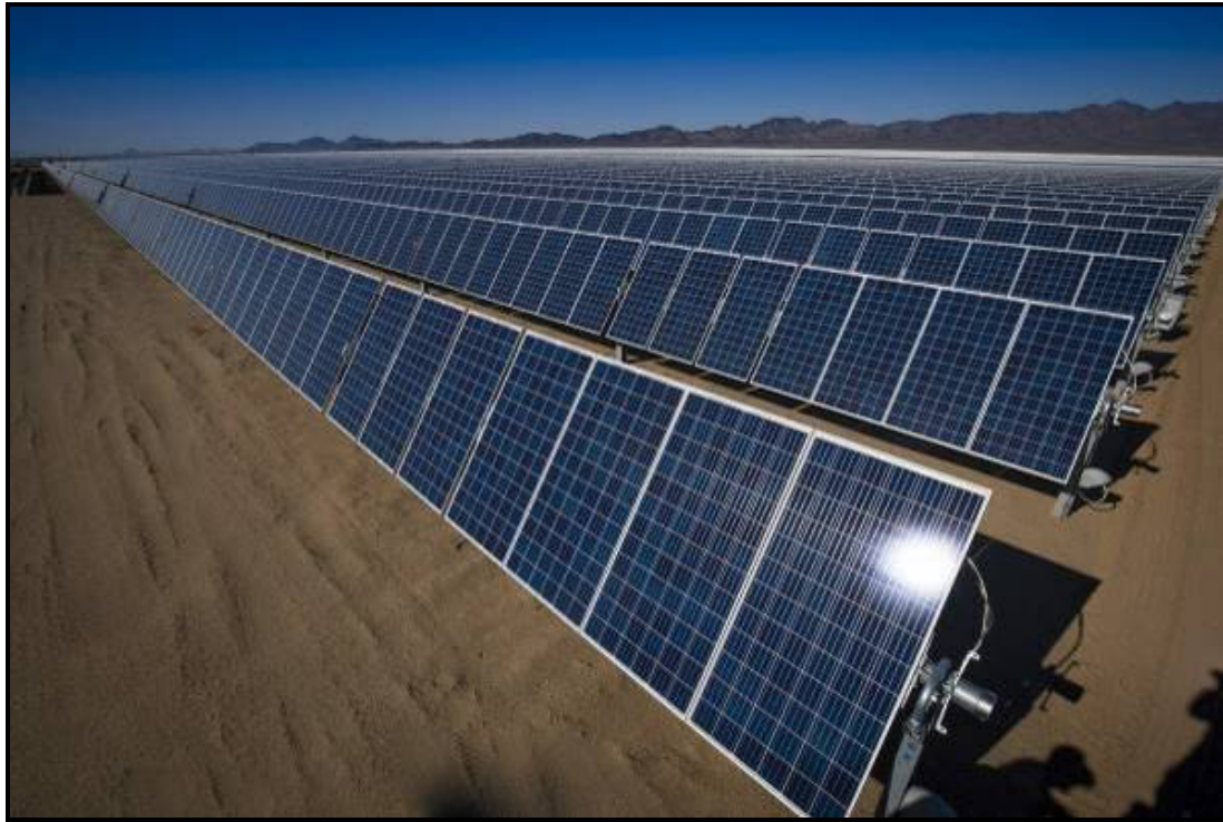
Photograph 1.1: Typical PV SEF facility
