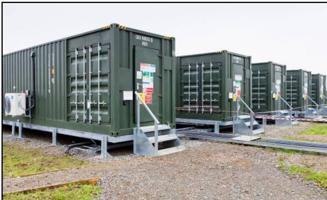
Photograph 1.2: Example of BESS located in storage containers
