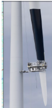
Figure 1: The single black-blade in the process of being painted in situ, at the Smøla Wind Farm. Painting white blades black after they are erected is more expensive than producing them at source.
