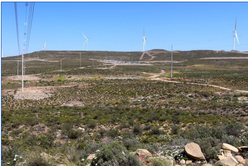
Figure 9: Region on De Hoop 202 just north of the Karusa WEF substation showing the extensive surface disturbance associated with the construction of even small powerlines.
