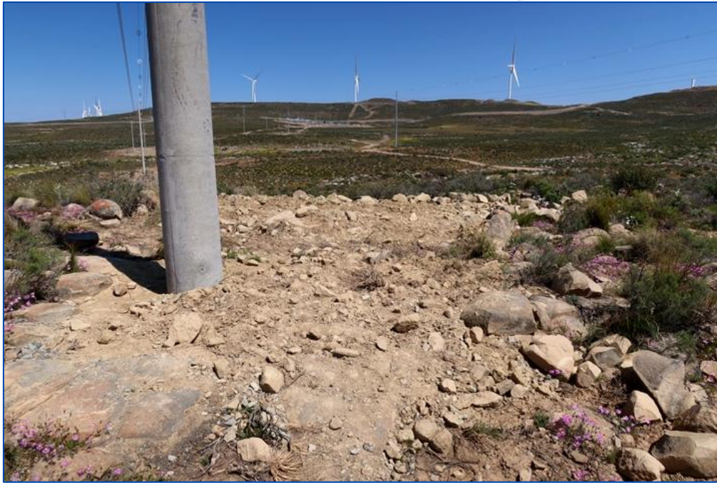
Figure 10: Close-up of a recently emplaced electrical pylon footing on the Karusa WEF. Recording of fossils within recently excavated rock rubble is rarely effective. Excavations for pylon footings are likely to have less impact on accessible fossil heritage than construction of the associated new access roads (see previous and following figures).
