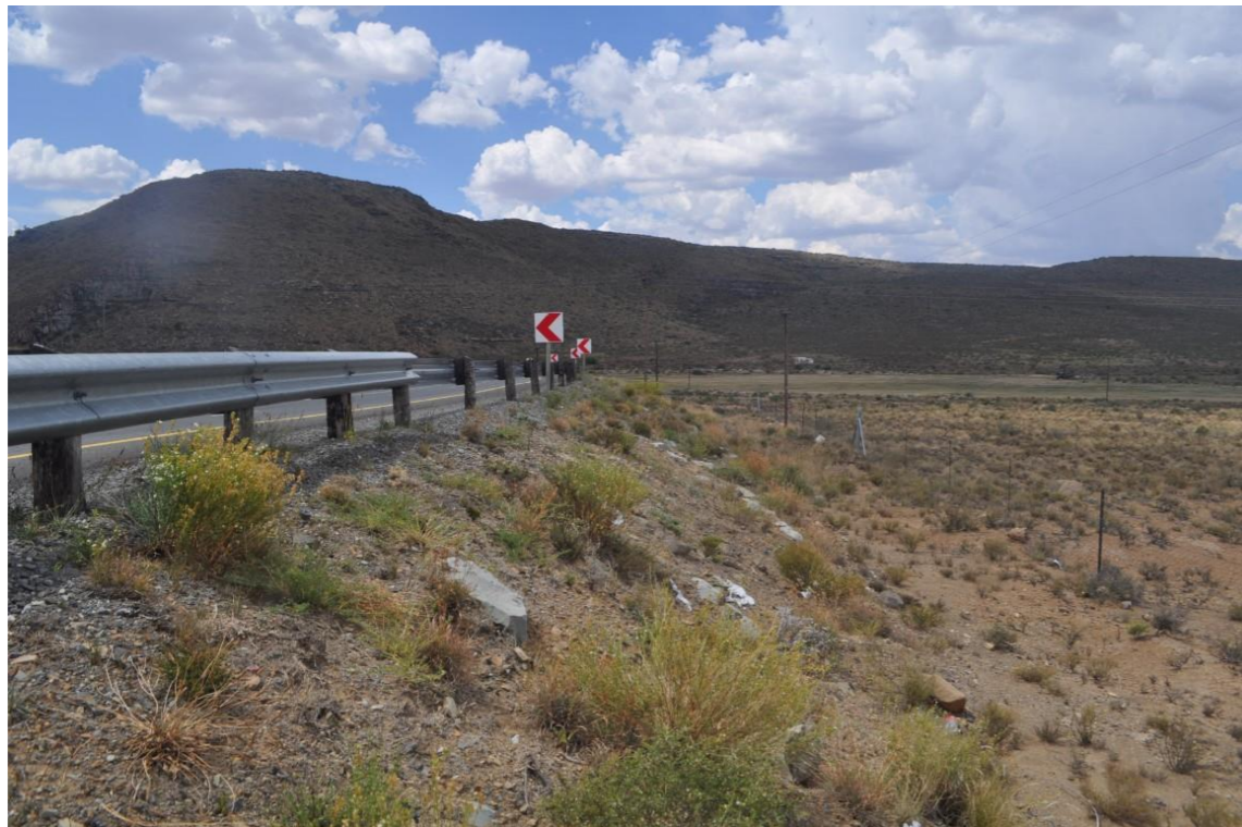
Road has been lifted / Guardrails / No Access to "road" shown on Google Earth
