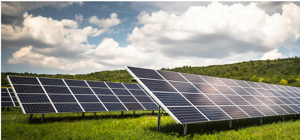
Figure 3-7: Fixed tilt system
