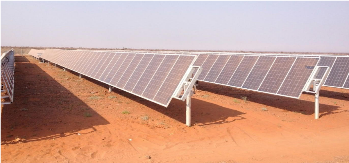
Figure 3-8: A single axis tracking system
