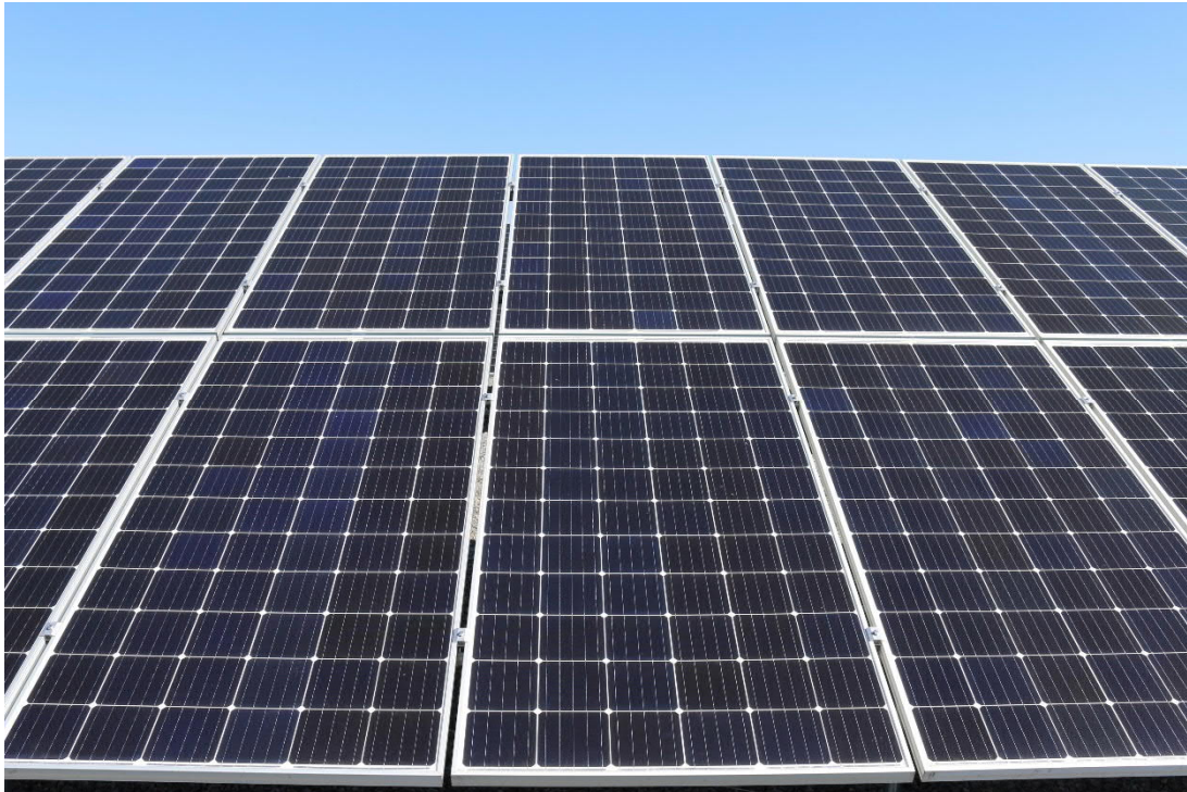
Figure 3-6 | Typical PV modules 7
