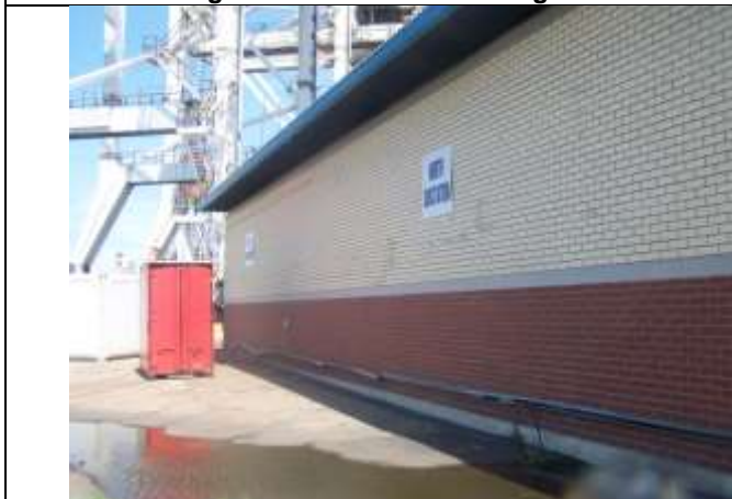
Image 5 – Existing North Substation
