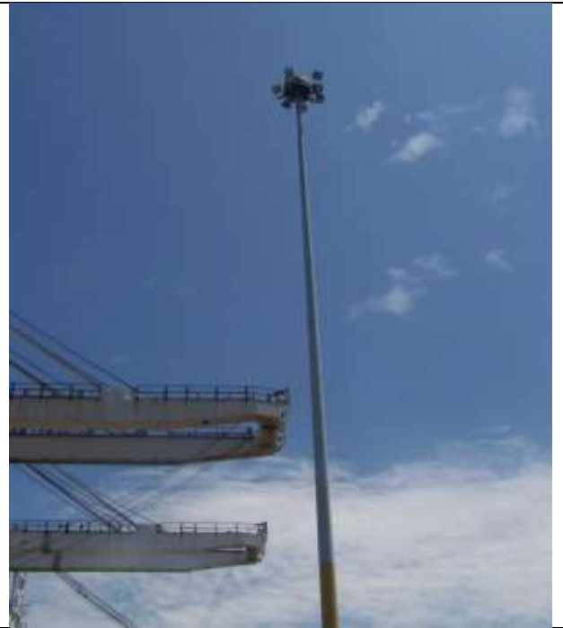
Image 4 – Existing High Mast Lights
