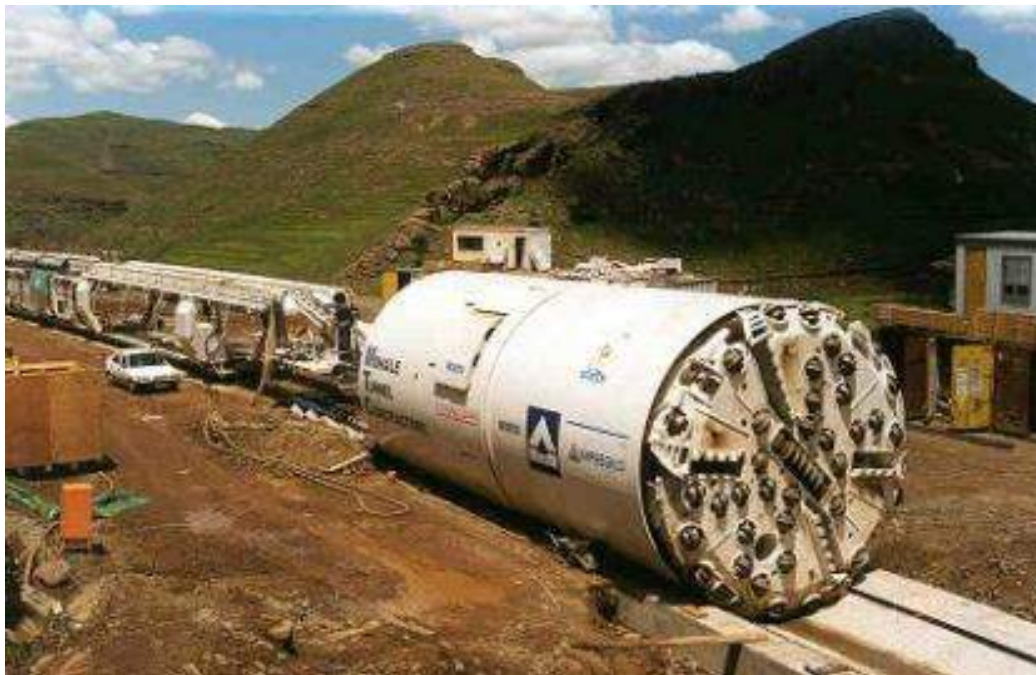
Figure 55: Example of a TBM ( http://www.tunnelforum.com/projects/?mode=type&id=3274 )
