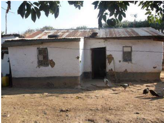
Lounge and two bedroom – Corrugated roof with mud walls Coordinates: 29°44'33.96"S – 29°54'32.83"E
