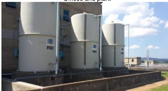
Poly flocculent storage tanks
