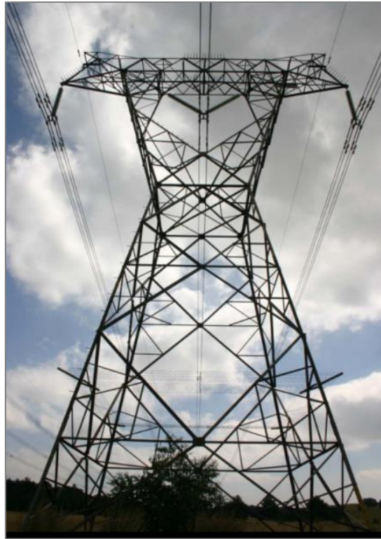
Figure 18: Tower Type 433A = Self Supporting Suspension tower
