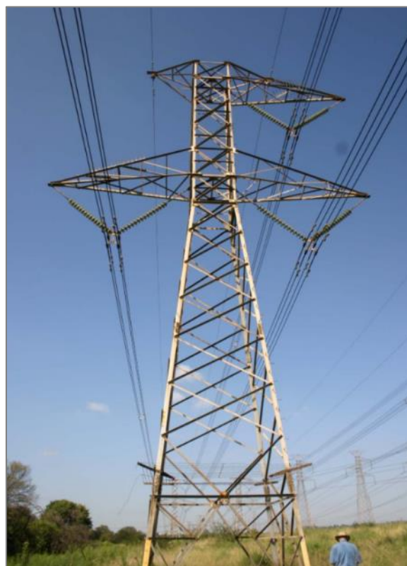
Figure 17: Tower Type 424 A - Self Supporting Suspension tower
