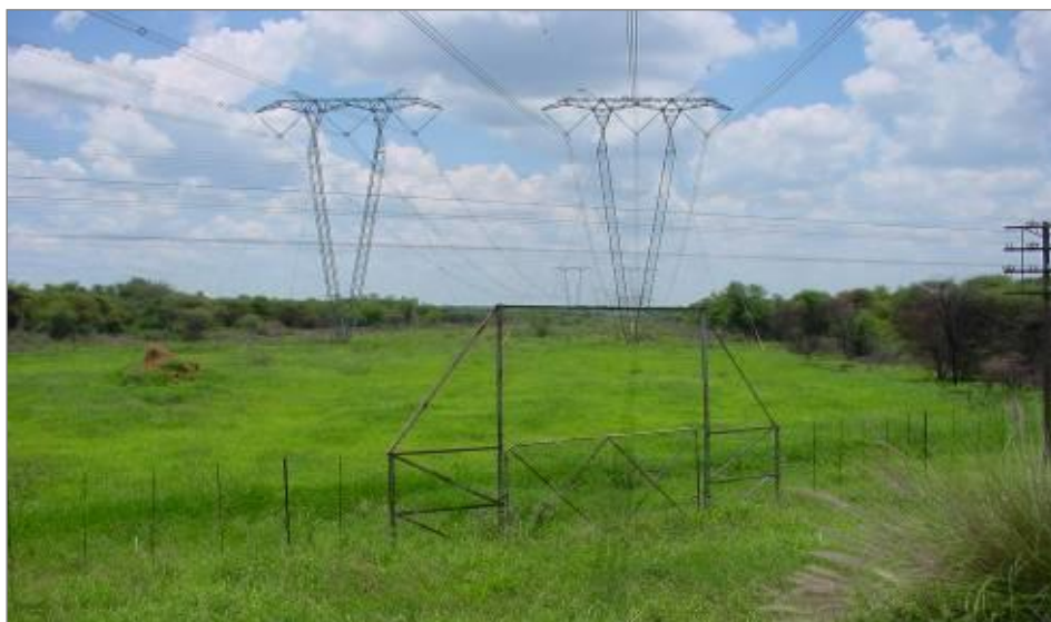
Figure 23: Access gate for an Eskom Tx line
