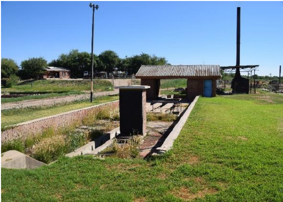
Figure 8: Obsolete “old” inlet works
