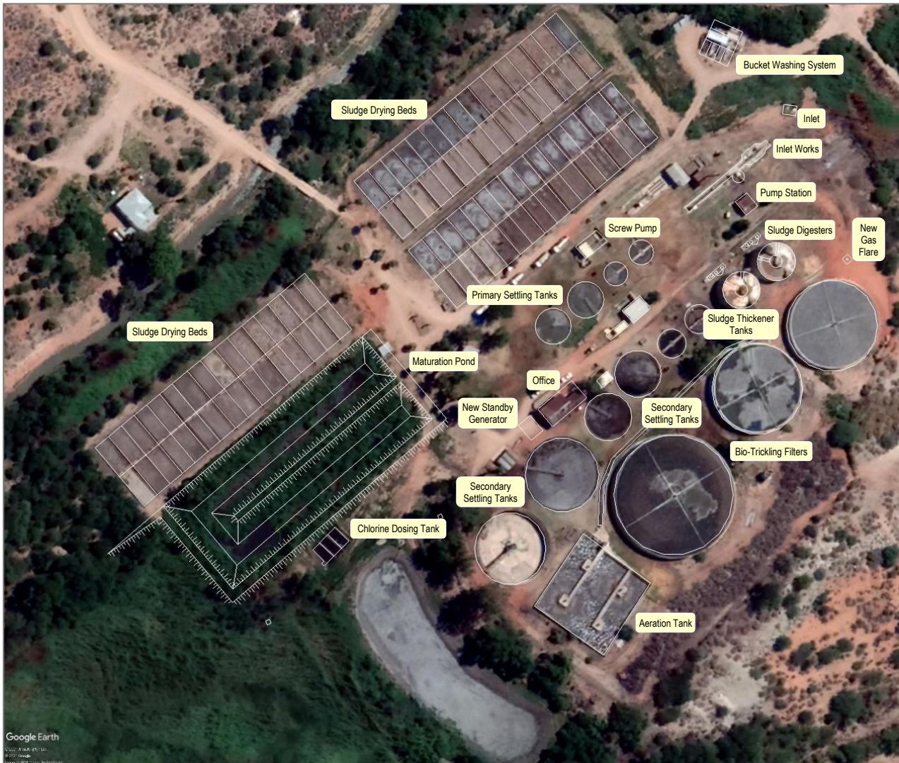
Figure 6: K-WWTW existing infrastructure to be refurbished (Google Earth image) (Not all infrastructure is labelled in the map above due to scale – see full details in map in Appendix D )
