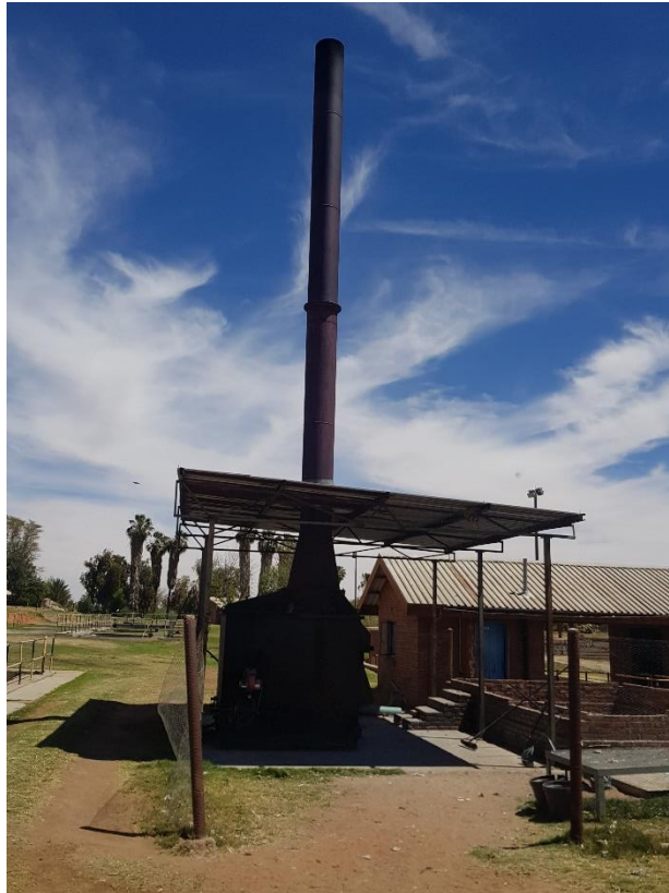
Figure 6: Existing incinerator at K-WWTW
