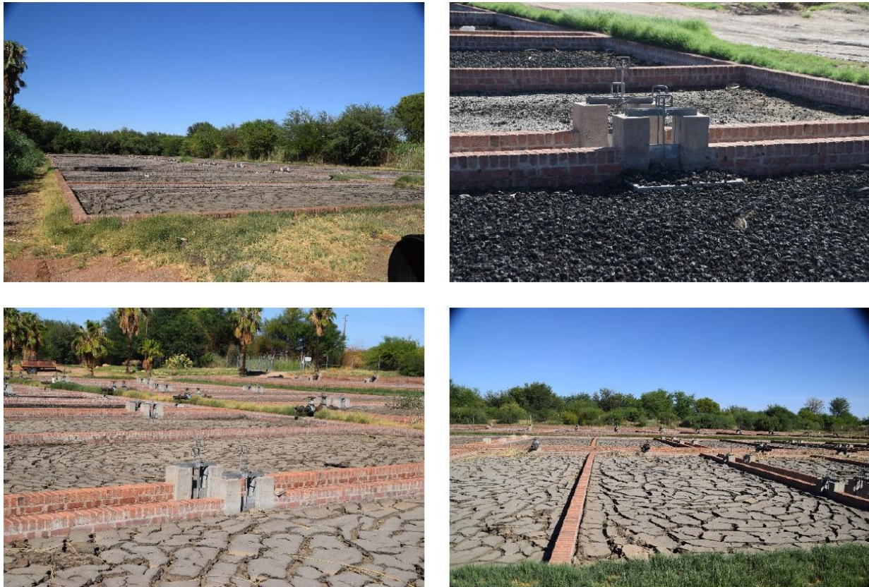
Figure 13: Sludge drying beds Set No 3 (top left), supernatant decanting Sets 1 & 2 (top right), Sludge drying beds Set 1 & 2 supernatant decanting (bottom left) and typical sludge drying bed (bottom right) (Bigen, 2020)
