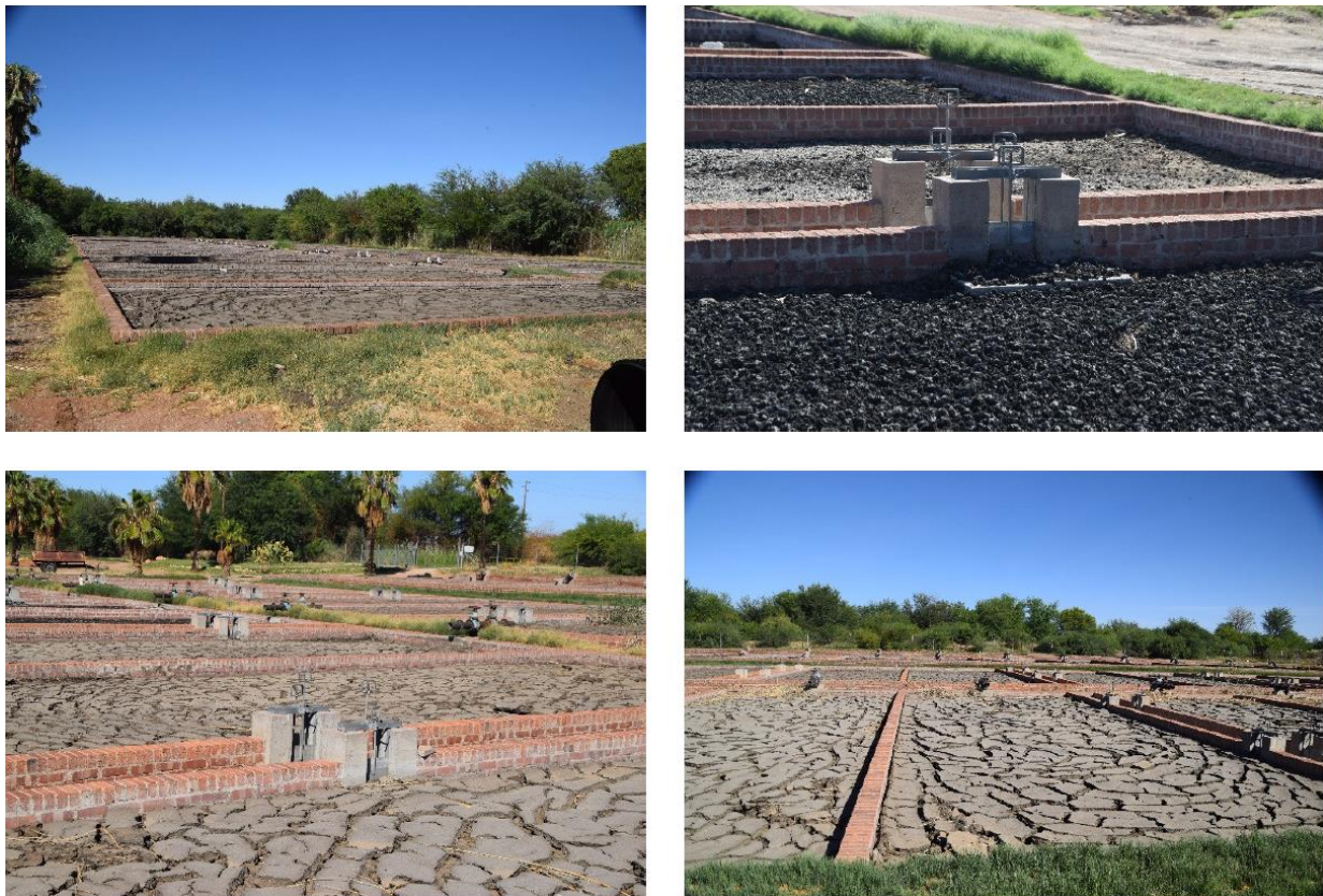
Figure 13: Sludge drying beds Set No 3 (top left), supernatant decanting Sets 1 & 2 (top right), Sludge drying beds Set 1 & 2 supernatant decanting (bottom left) and typical sludge drying bed (bottom right) (Bigen, 2020)
