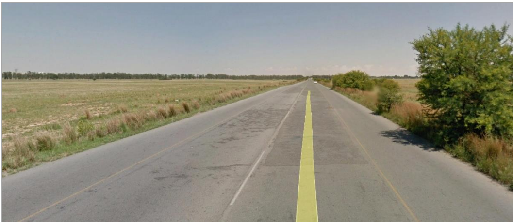
Figure 48: North-western view along the R70 (primary site located to the left) (Google Earth image)
