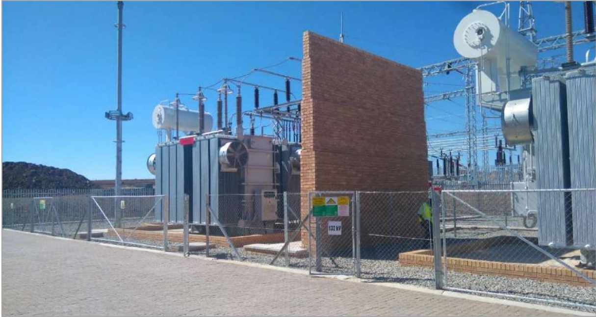
Figure 16: Example of High Voltage Transformers
