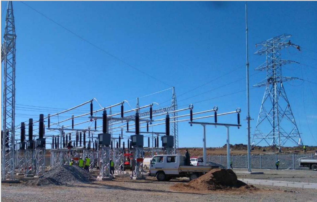
Figure 23: Example of High Voltage Transmission Line Connecting to Substation
