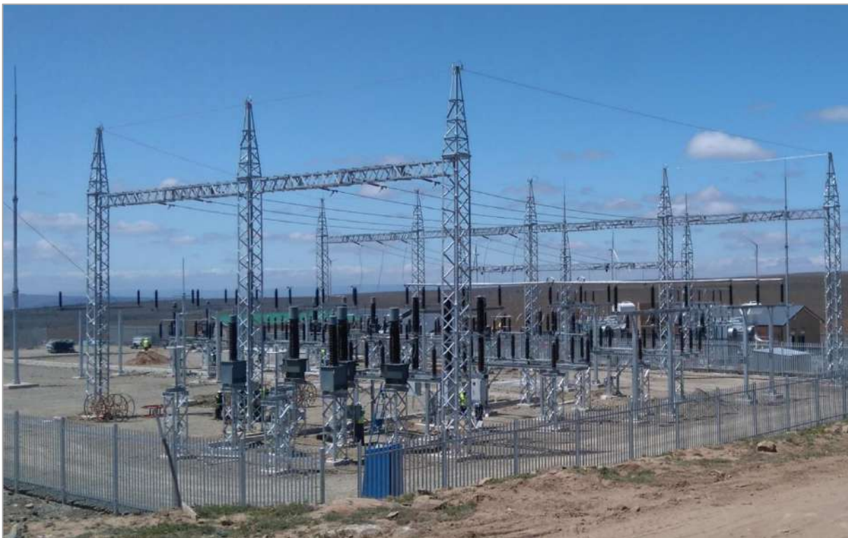
Figure 15: Example of High Voltage Substation
