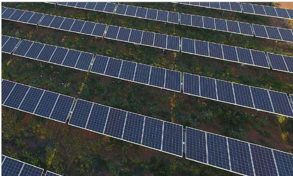
Figure 13: Example of Rows of PV Modules Mounted on Single Axis Trackers from PIA Solar
