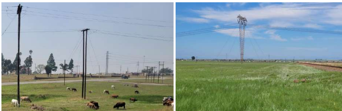
Figure 68: View of overhead services in Leandra (top) and surrounding rural areas (bottom)
