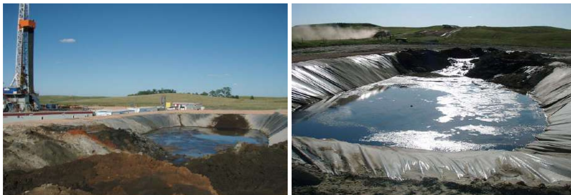
Figure 87: Examples of pits used to separate cuttings from drilling fluids (by Joshua Doubek - Own work, CC BY-SA 3.0, https://commons.wikimedia.org/w/index.php?curid=27167604 )
