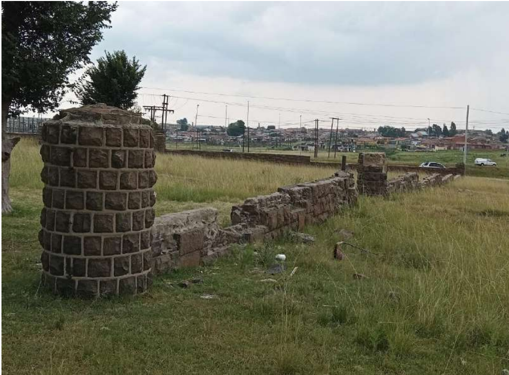
Figure 60: View of the surrounding wall, built from dolerite stone, showing one of the circular pillars
