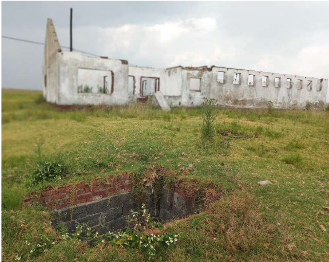
Figure 73: View of the long rectangular structure, showing a brick cistern or cellar in the foreground
