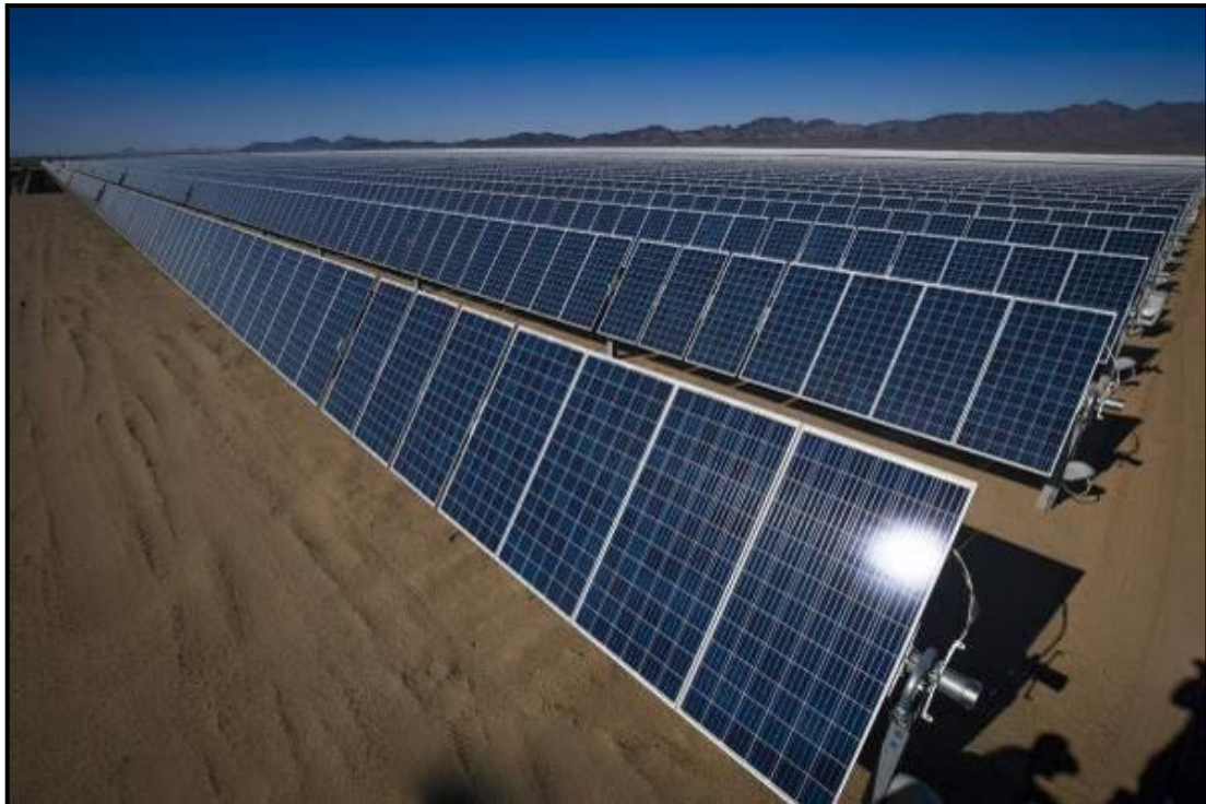
Photograph 1.1: Typical PV SEF facility
