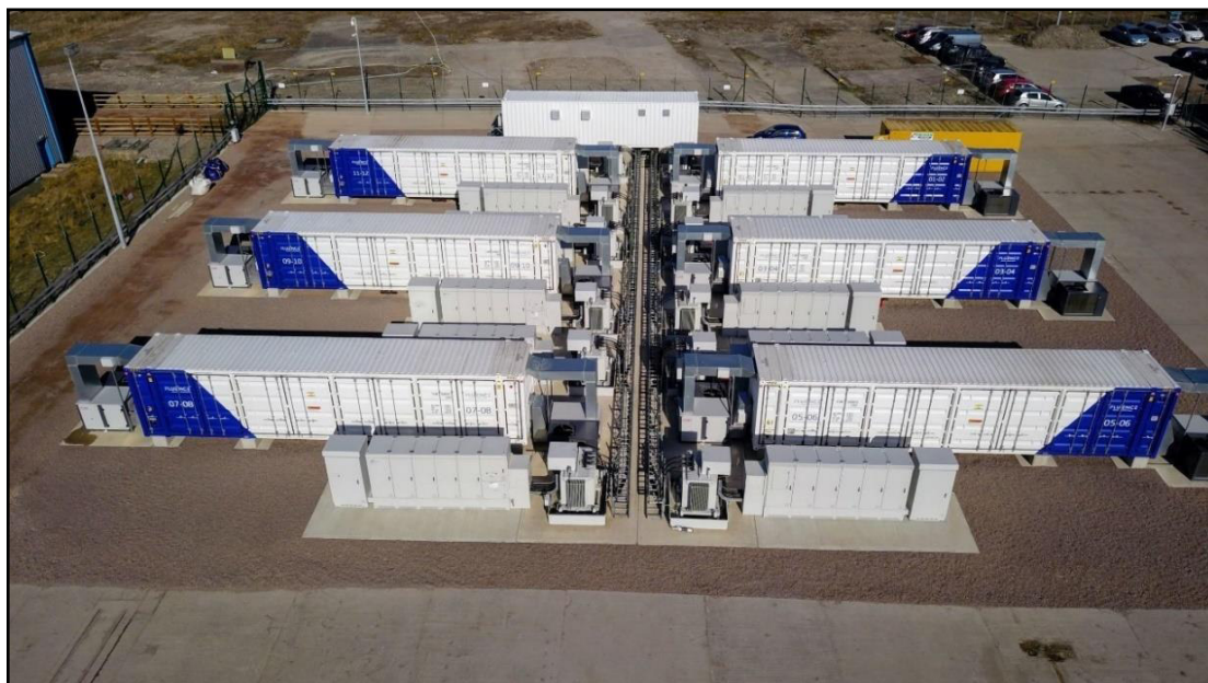
Photograph 1.2: Example of BESS located in storage containers
