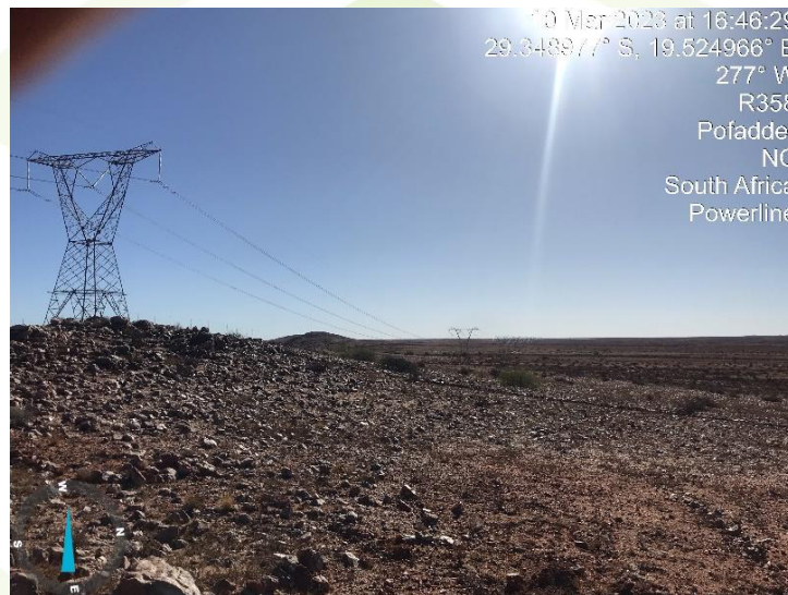
Figure 4.10: Powerline viewed from the R358
