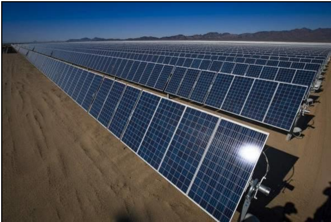
Figure 1.2: Typical PV SEF facility
