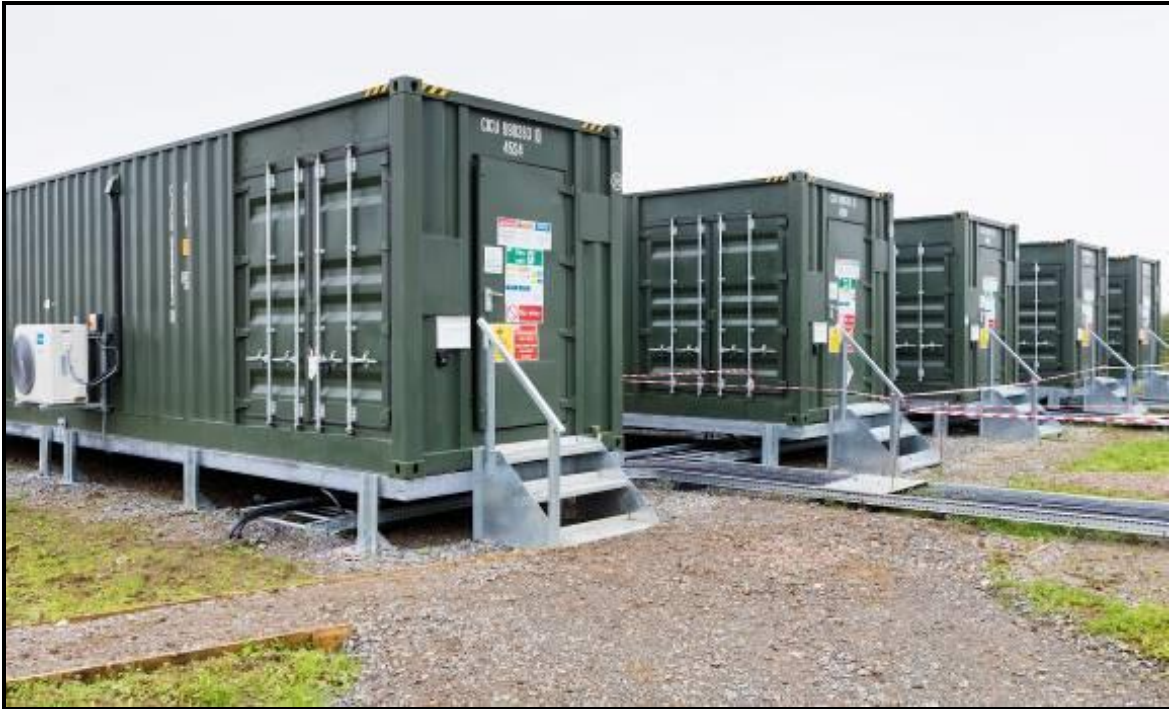
Figure 1.3: Example of BESS located in storage containers
