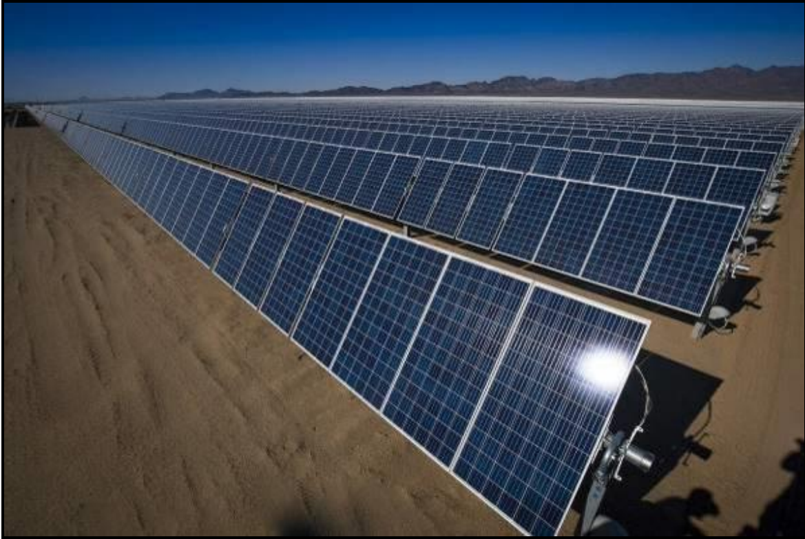
Figure 1.2: Typical PV SEF facility
