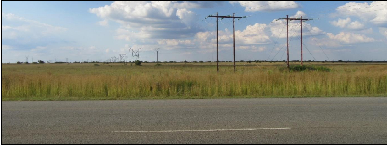
Photograph 3.10: 88 kV lines traversing the R305 on Elandsfontein 34/7.
