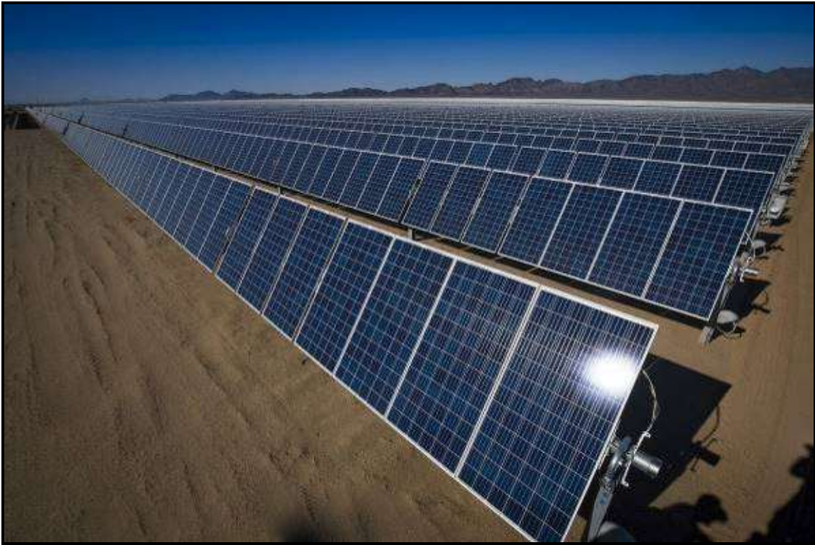
Figure 1.2: Typical PV SEF facility
