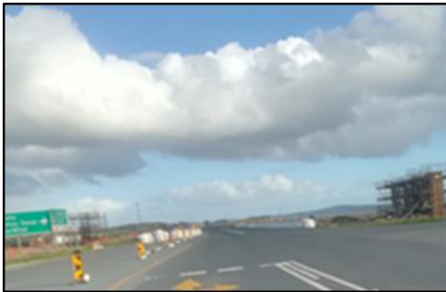
Pic 3 - West East orientated road intersection with R27 near old Weighbridge (note new interchange in construction to connect west-east orientated link road to the R45)
