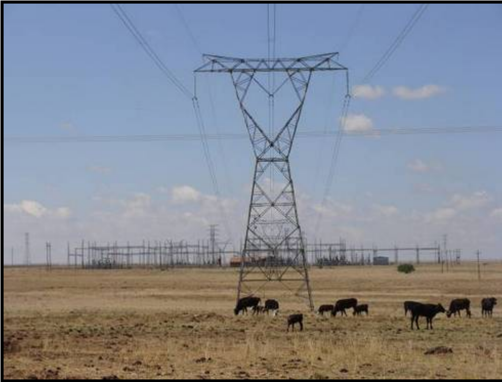
Photograph 3.4: Power lines running south from the Merapi substation
