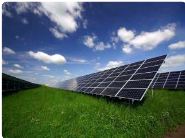
Figure 2: Picture of a PV Panel (Courtesy of Decchi)
