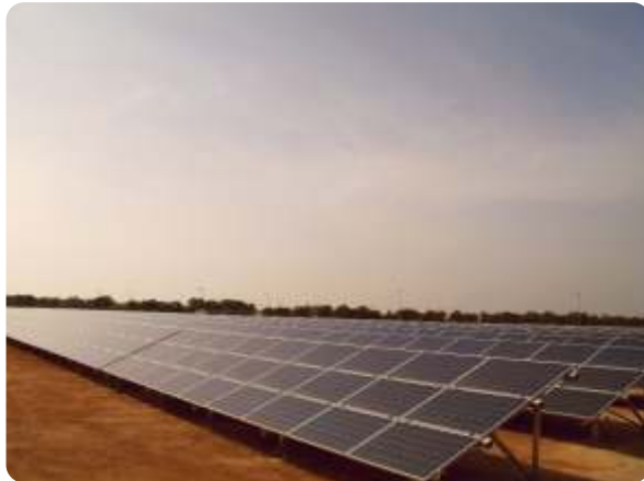
Figure 2: Picture of a PV Panel ( http://www.frv.com/multimedia-files/ )
