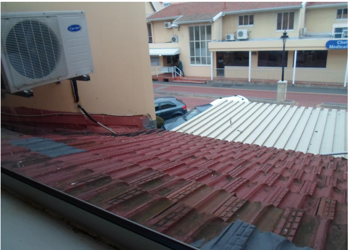
Image 8: View from within the St Augustine's Medical Centre 2 looking out over the roof of the entrance.
