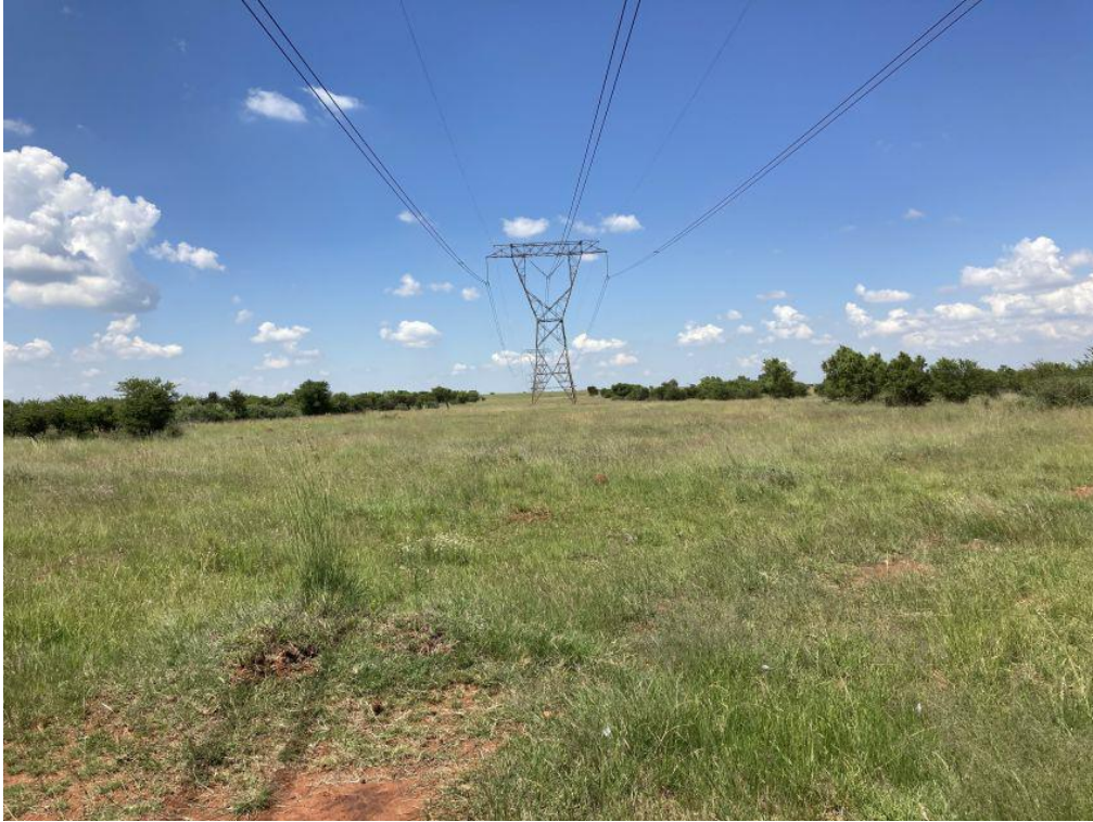
Figure E8: High voltage overhead powerline in the proposed development area.
