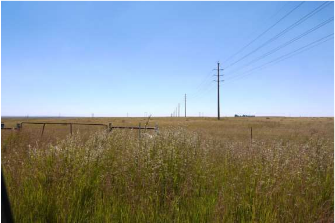
Plate 16 - A view along the line of a 132kv overhead power line with monopole towers
