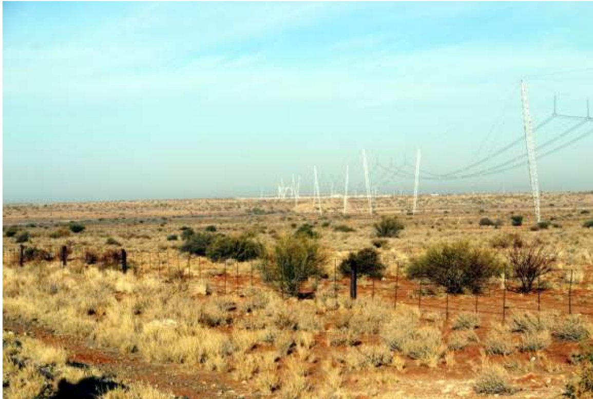
Plate 1, Existing Upington Main Transformer Substation (MTS). Note strategic power line connections linking to the MTS
