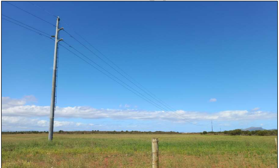
Figure 3: Photographic example of monopoles structure ( Source VRM Africa Lundskip VIA)
