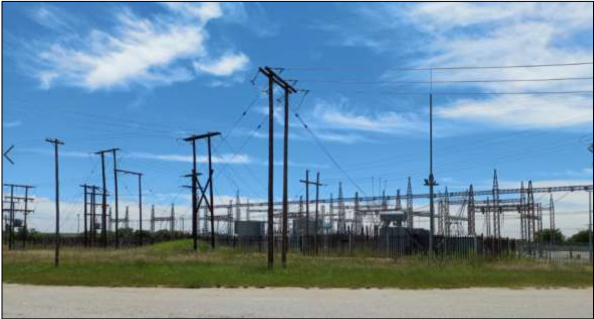
Figure 12: Photograph of Rietkuil Substation.
