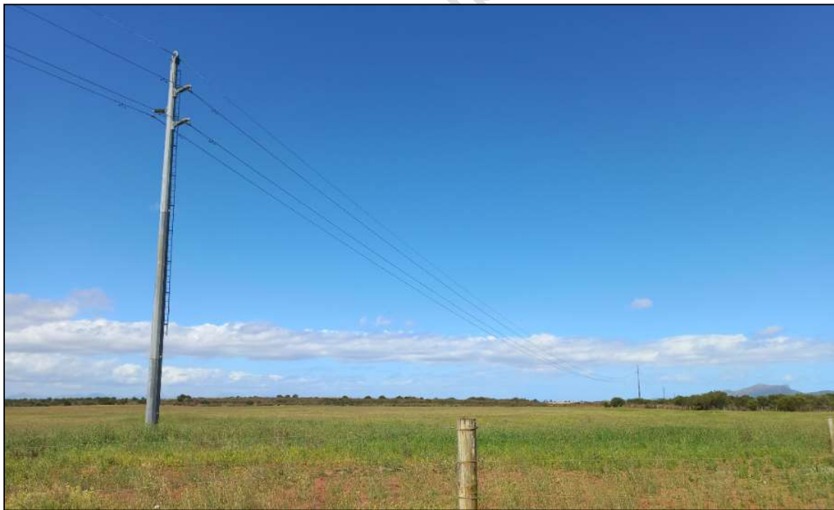
Figure 3: Photographic example of monopoles structure ( Source VRM Africa Lunskip VIA)
