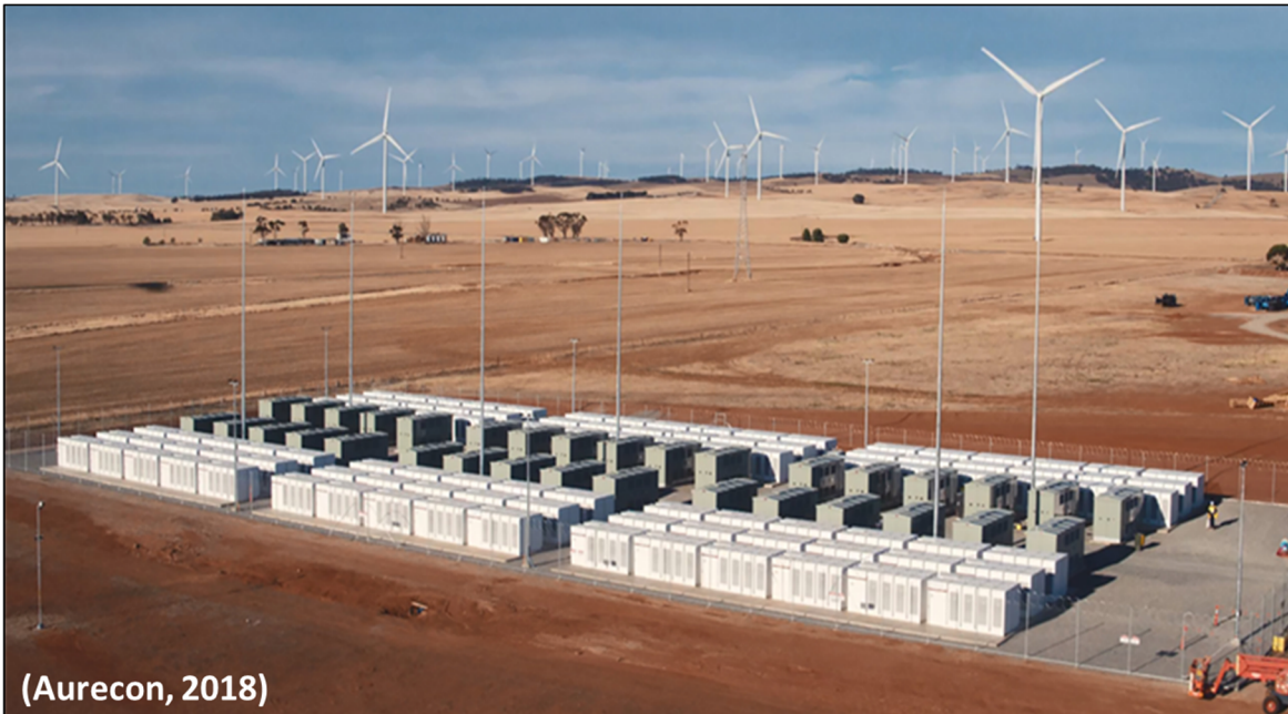
Figure 2: The 100 MW/129 MWh Li-ion battery coupled with the Hornsdale wind farm in Australia.
