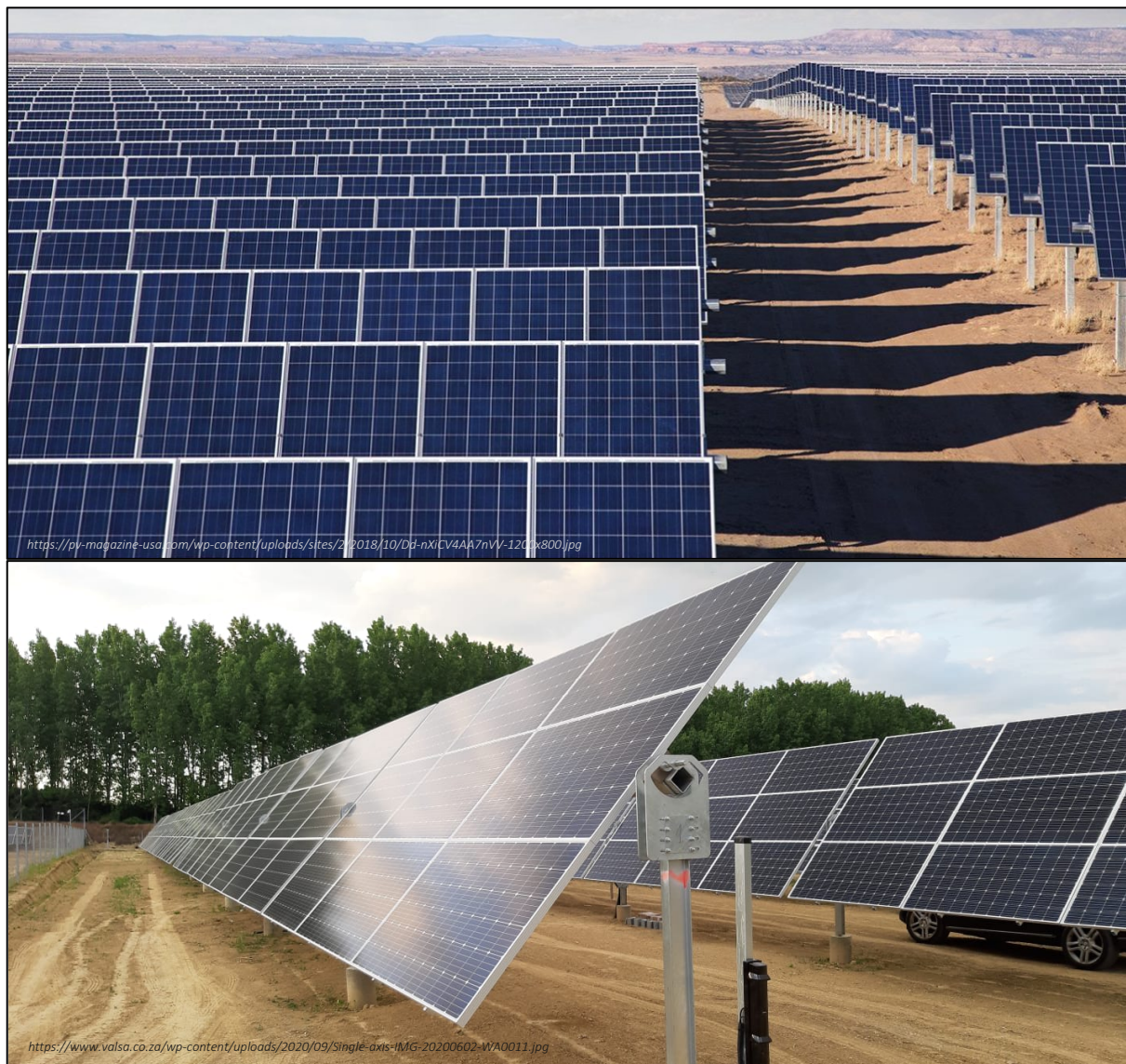
Figure 3.3 – Examples of installed PV systems
