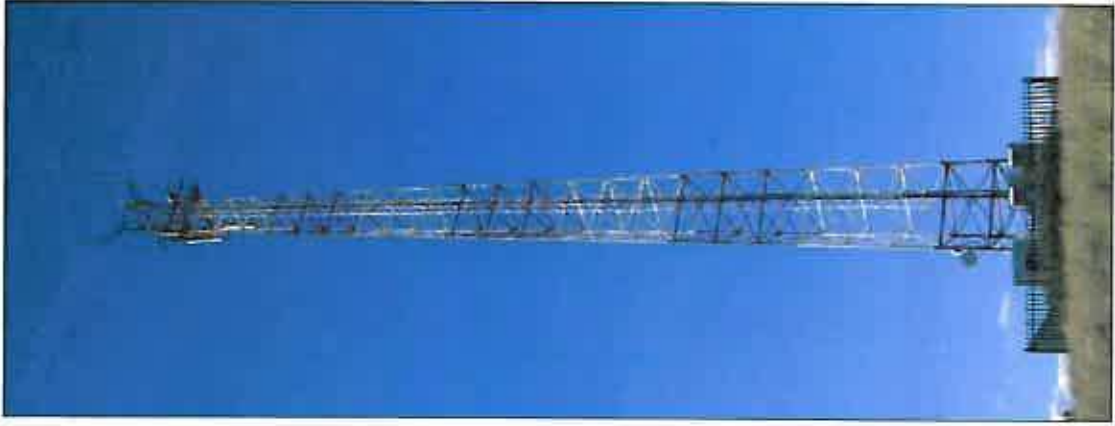
TYPICAL 3-LEGGED LATTICE MAST (PAINTED RED & WHITE)
