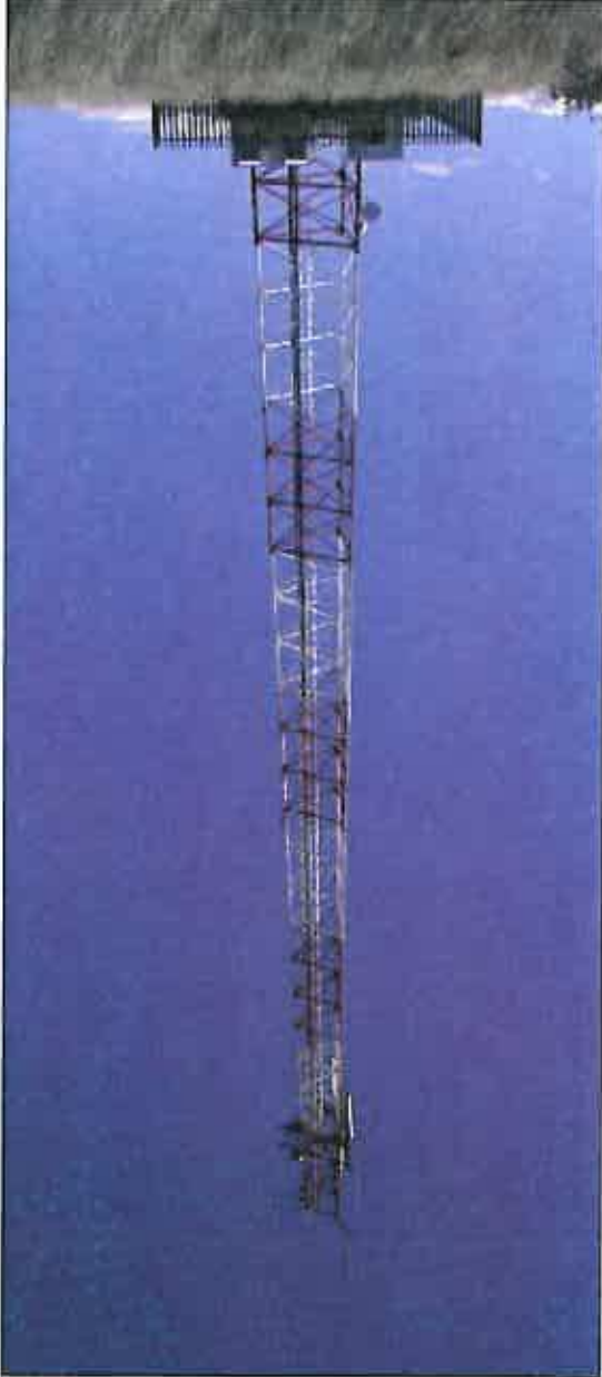
TYPICAL 3-LEGGED LATTICE MAST (PAINTED RED & WHITE)
