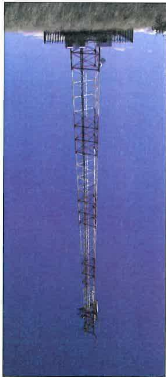
TYPICAL 3-LEGGED LATTICE MAST (PAINTED RED & WHITE)
