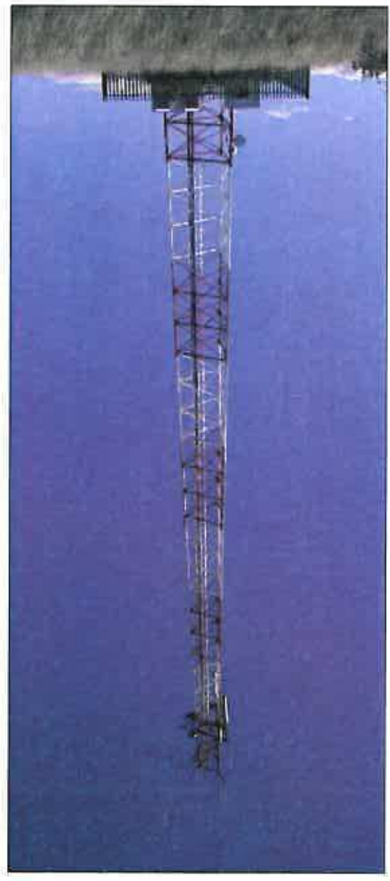
TYPICAL 3-LEGGED LATTICE MAST (PAINTED RED & WHITE)
