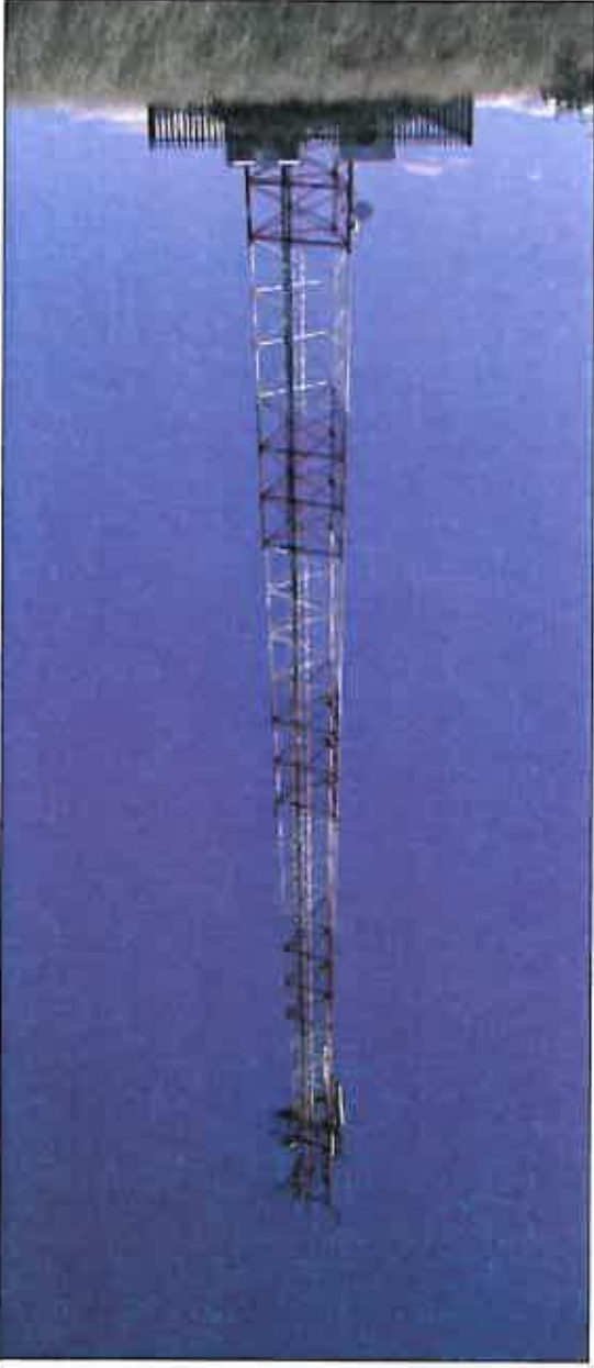
TYPICAL 3-LEGGED LATTICE MAST (PAINTED RED & WHITE)
