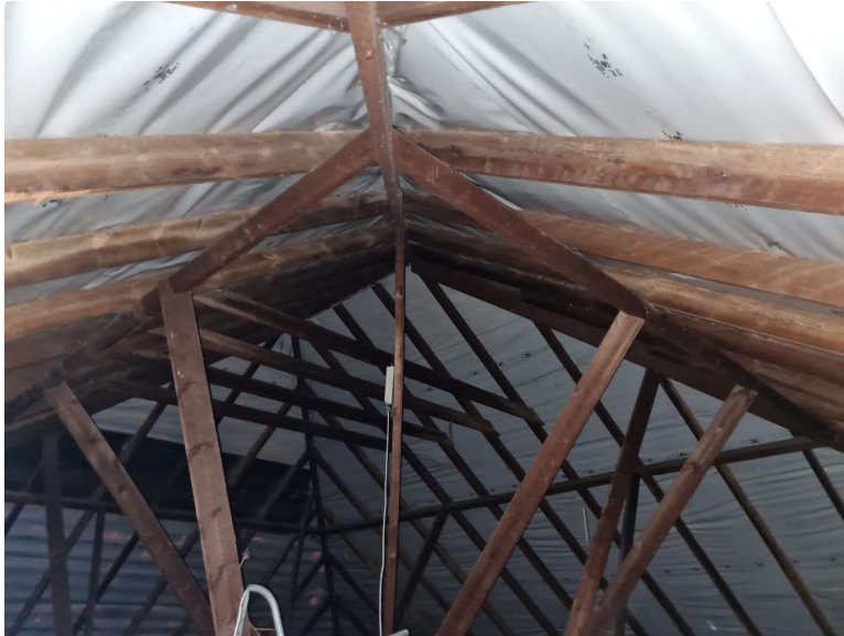
MAIN DWELLING – EVIDENCE OF WOOD BORER INFESTATION IN CEILING VOID
