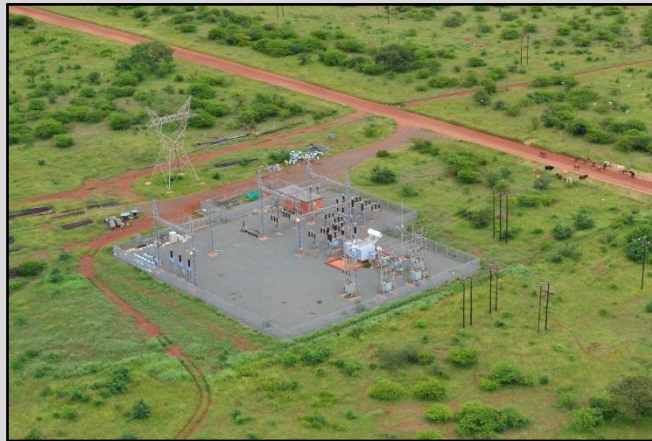
Figure 1: Typical Photo of a similar sized Substation
