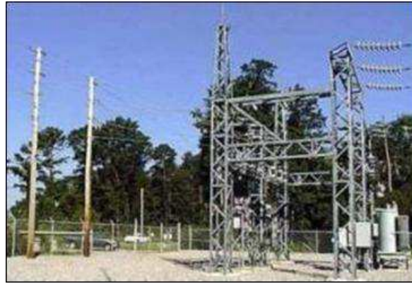
Figure 5-4: Distribution bus and low voltage distribution power lines.
