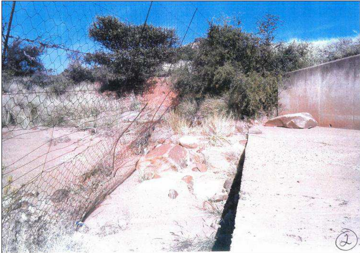
Figure 7-14: Erosion occurring where concrete structures ends on farm Lupani (Foto courtesy of D. Ford).
