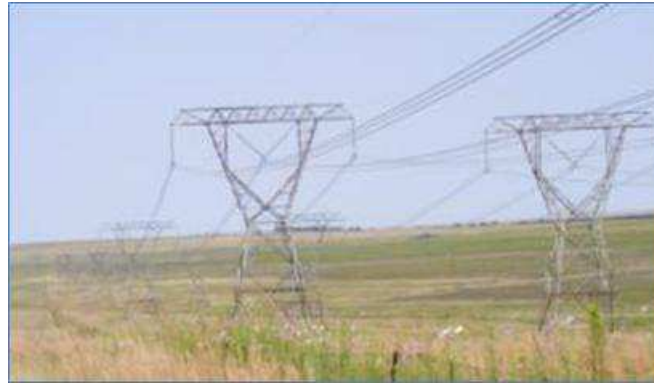
Figure 5-2: Typical transmission power lines.
