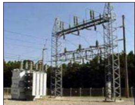
Figure 5-3: Example of a transformer, incoming power from the transmission grid, a set of switches for the incoming power and distribution bus plus three voltage regulators.
