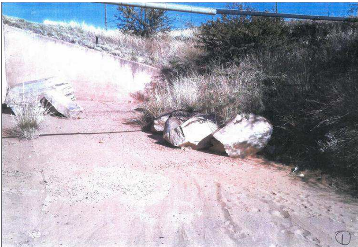
Figure 7-13: Erosion along the water courses on the farm Lupani where a bridge has been built (Foto courtesy of D. Ford).
