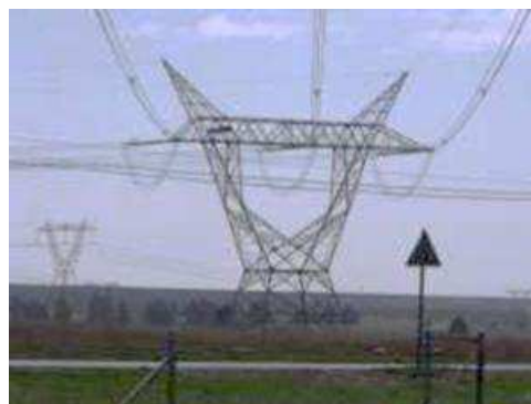
Figure 1-3: Example of 400 kV Tower.
