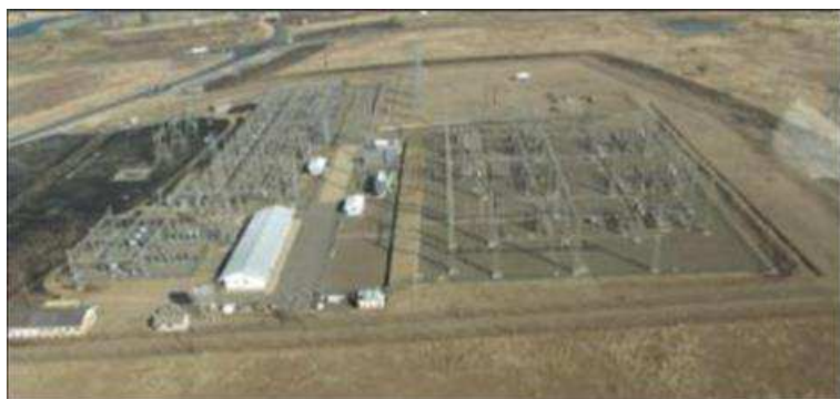
Figure 1-4: Example of a substation.
