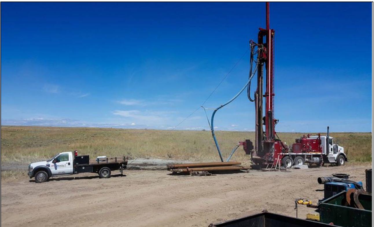
Figure 3: Example of the type of drilling rig to be used. Source: Basic Assessment Report Figure 4.
