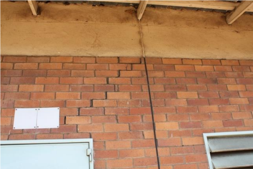
Figure 8: Example of blast induced damage.
