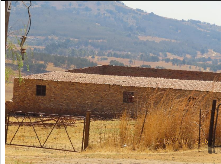
Old Brick and Mortar Structure (with damage)
