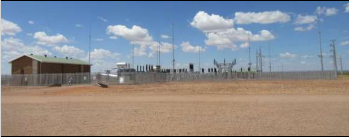
Photograph 3.10: Daysonsklip 1&2 SEF substation and 132 kV line on Dayson's Klip
