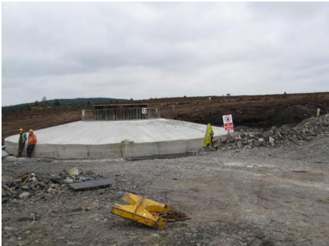
Figure 13: Example of the construction of the foundation of a single wind turbine (UK Department of the Environment and Northern Ireland Environment Agency, 2015)
