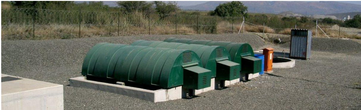
Figure 3-4: Typical example of WWTW
