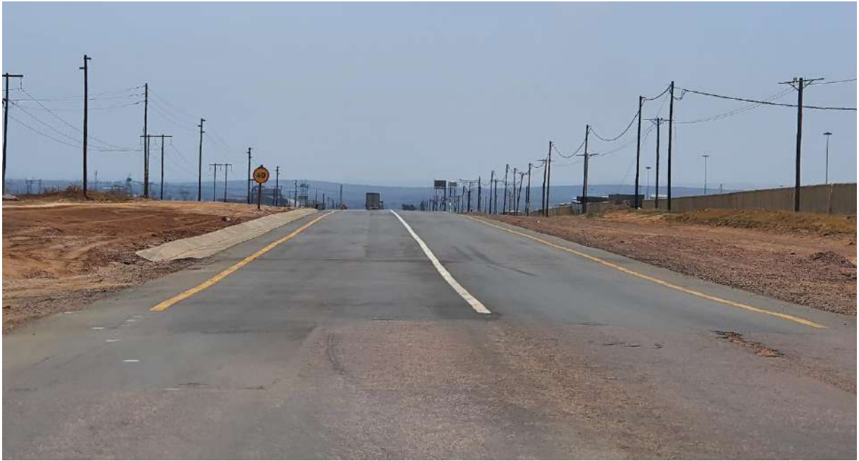
Photo 2: Looking north along the N11 leaving the N4 interchange approaching the resurfaced area
