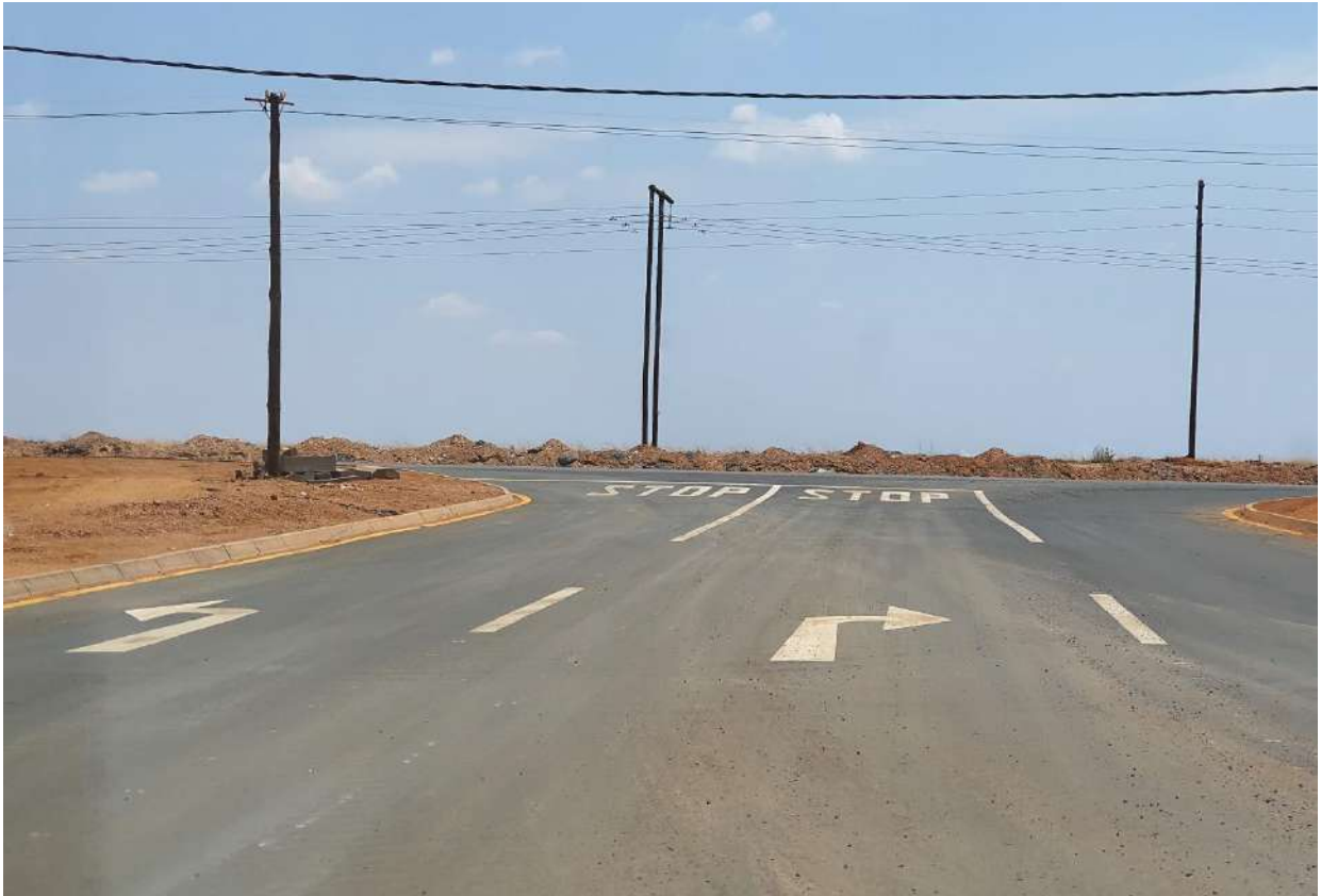
Photo 10: Looking west along Road D at the N11 (recently constructed new intersection adjacent the Site which on the right).
