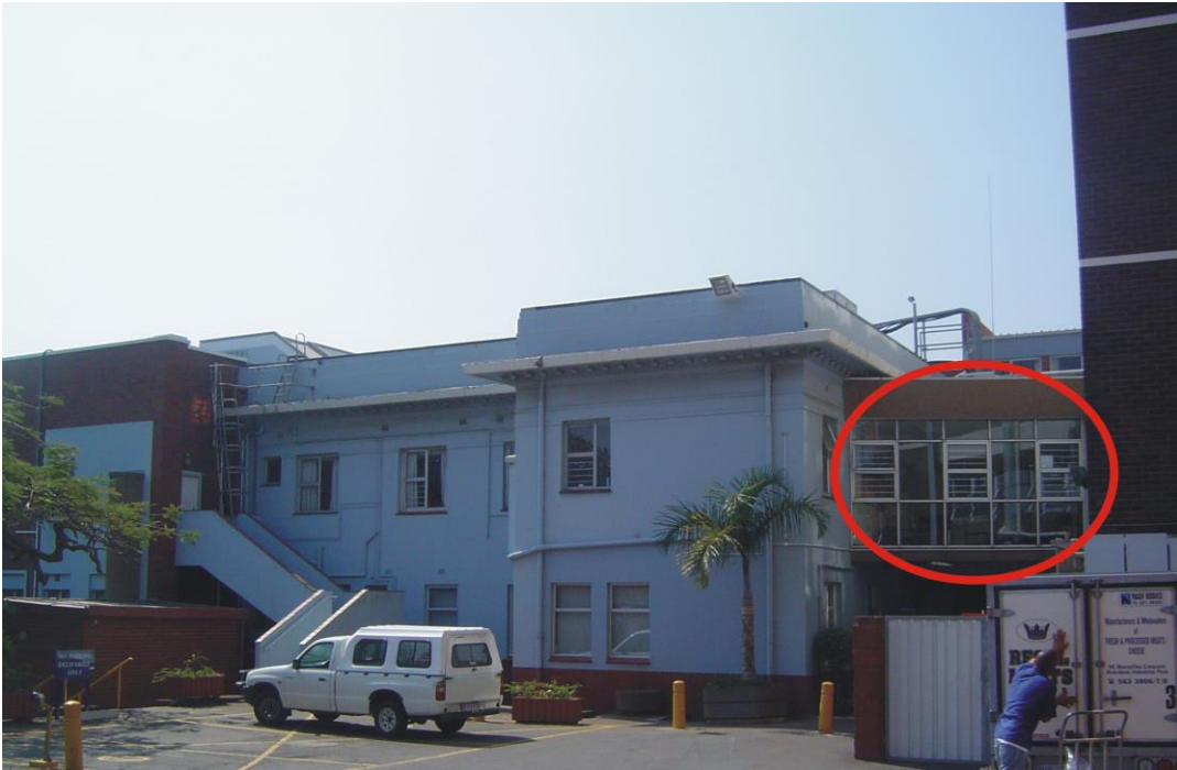
Photo 3: Existing façade and staircase of existing neurology ward. Existing link passage shown (red) – this façade is proposed to be demolished to provide a new link passage to the proposed twenty bed ward and existing hospital.
