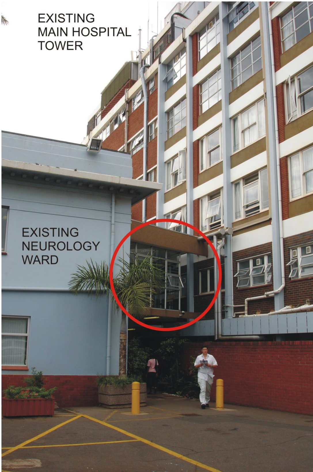
Photo 5: Existing façades and link passage (red) of neurology ward and the existing hospital tower.
