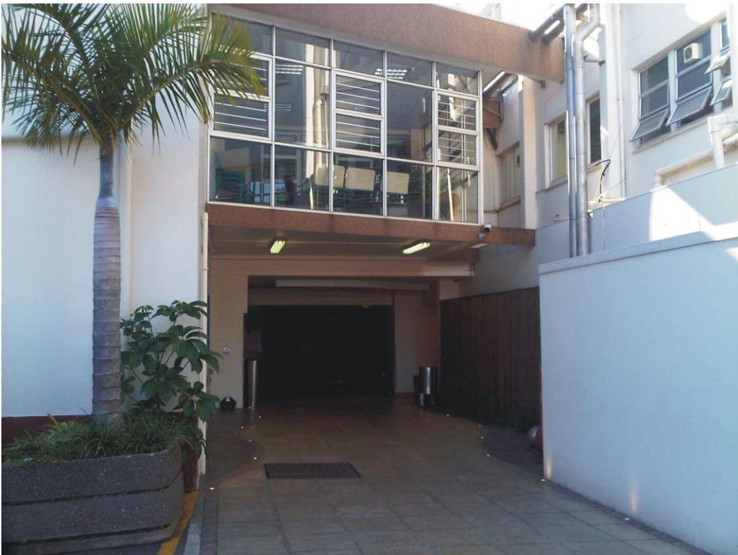
Photo 4: Existing link passage façade which will be demolished to create the new link passage from the proposed twenty bed ward to the existing hospital.
