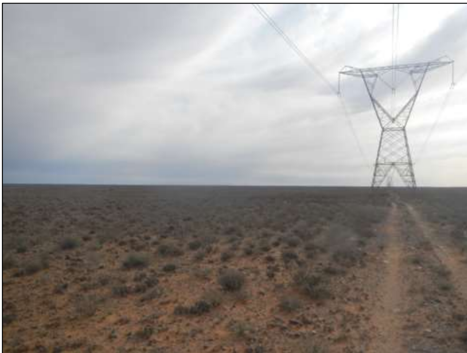
Figure 56: View of the existing power line and servitude which power line corridor option 2 is aligned to follow
