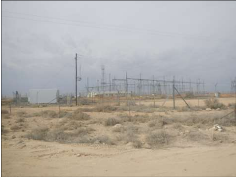
Figure 55: View of the existing Eskom Kronos Substation
