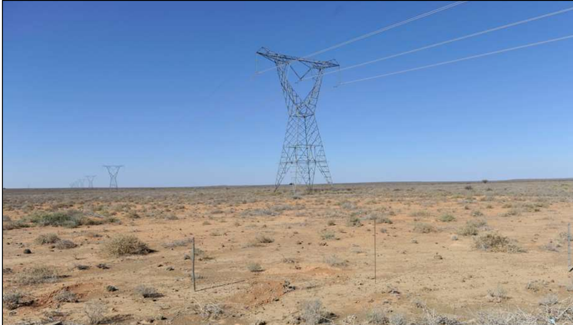
Figure 18: The existing Aries-Kronos 400kV transmission line which runs just south of the proposed development site.
